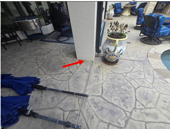
Inadequate clearance/drainage at columns.
