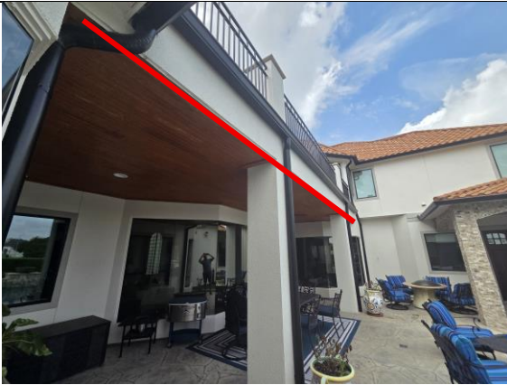
No drainage provision under rear balcony soffit. NOTE: No elevated moisture readings in area.
