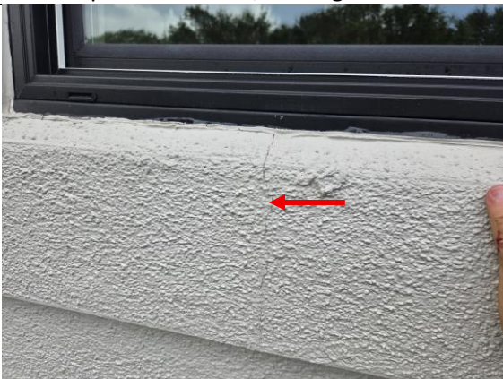
Minor crack at left elevation trim band.
