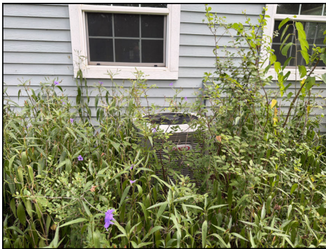
Heavy foliage observed at the garage apartment condenser unit
