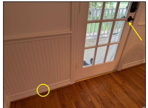
Doorstop noted to be missing at the dining room exit/hardware is installed upside down
