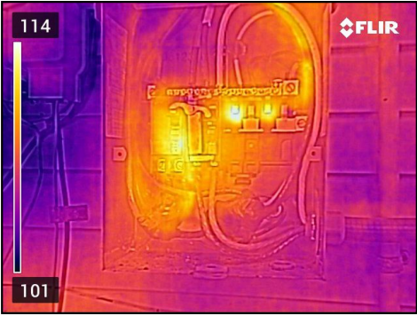
Panel appeared to be performing as intended
