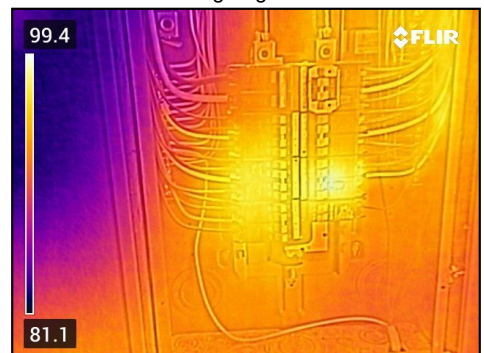
Panel appeared to be performing as intended
