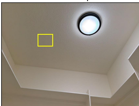
Supply duct was not present inside the kitchen pantry
