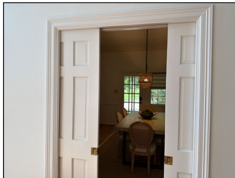
Dining room pocket doors were difficult to operate
