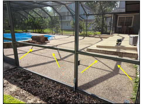
Deteriorated screen material observed at the rear enclosure/Loose spline observed
