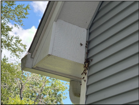
Aggressive paper wasps observed at the front left of the home/Inspector was stung walking the roof
