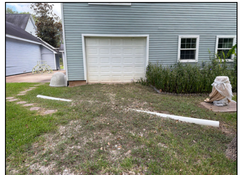
Grading is less than ideal at the garage apartment
