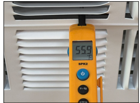
AC supply temperature/Units were cooling well at the time of inspection
