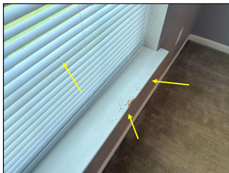
Damaged window stool trim observed at the garage apartment
