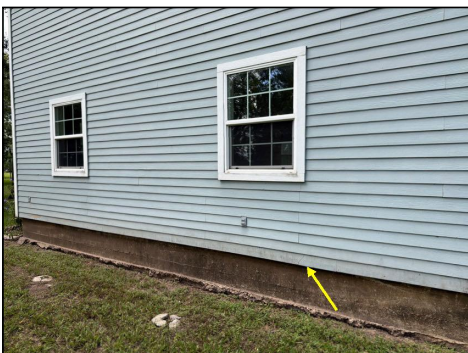
Damaged siding observed at the garage apartment
