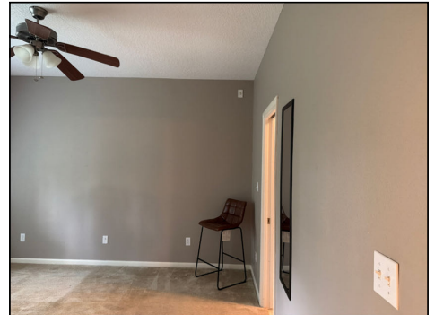
Ceiling fan/light did not function at the garage apartment
