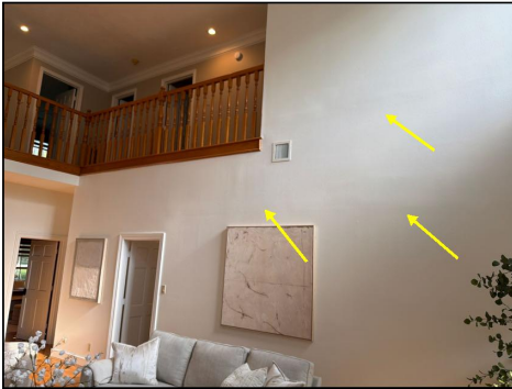
Poor drywall finish/visible seams observed at the family room
