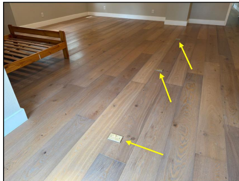
Floor plugs in the right rear game room are not flush to the floor/trip hazards
