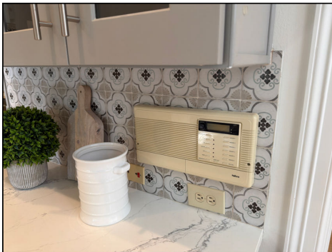
Intercom system was not inspected
