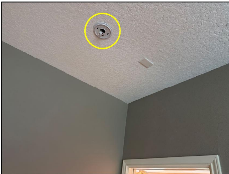
Smoke alarms noted to be missing throughout the garage apartment
