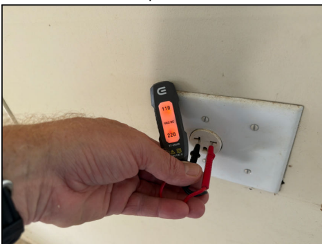
220 outlet at rear garage appeared to be performing as intended
