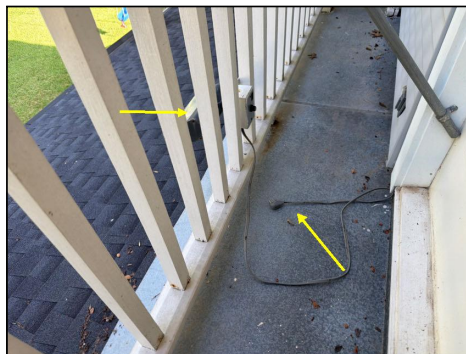
Out of ordinary exterior fixture observed at the front balcony/removed from service
