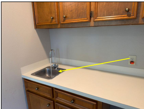
Wet bar outlet is not GFCI protected
