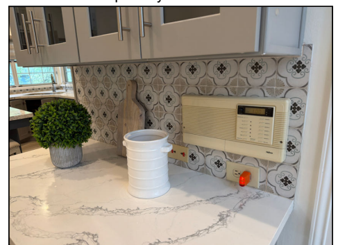
Kitchen backsplash outlet is not GFCI protected/spacing does not meet current standards
