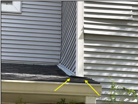
Raised flashing observed on the right side of the home
