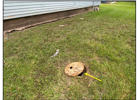
Cover for subsurface propane tank is less than ideal/loose
