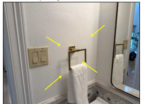
Missing/inconsistent wall texture observed in the half bathroom
