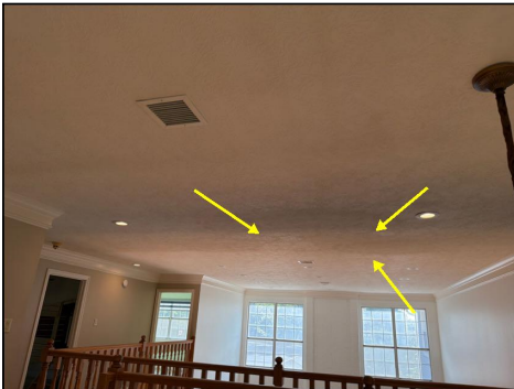
Inconsistent finish/evidence of previous repairs observed at the ceiling above the family room
