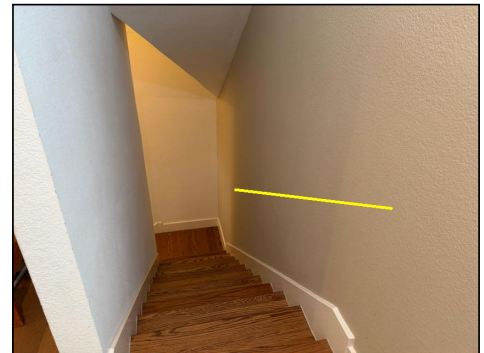
Handrail noted to be missing at the rear stairs
