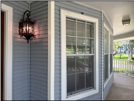
Exterior walls noted to be dirty around the perimeter of the home
