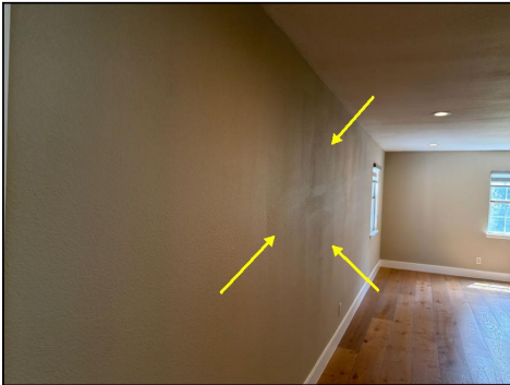
Poor quality drywall/paint finish observed at the upstairs right rear room
