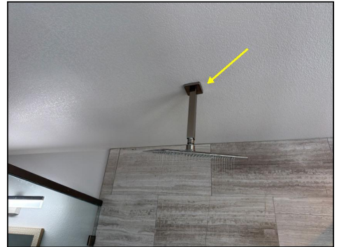
Upstairs right overhead shower line is loose behind the drywall
