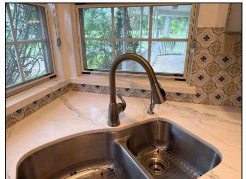
Water pressure down to trickle at some times during inspection
