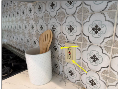
Kitchen backsplash outlet is not installed properly
