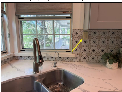
Switch at the kitchen sink noted to be abnormally high
