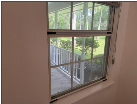
Interior primary bedroom window would not open
