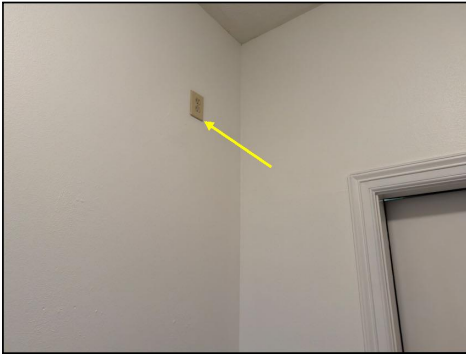
Out of ordinary outlet placement observed in the laundry room
