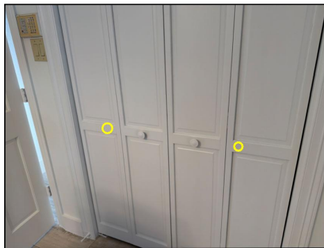
Hardware at the breakfast area closet doors is not installed properly
