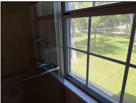
Less than ideal configuration at the left secondary shower surround
