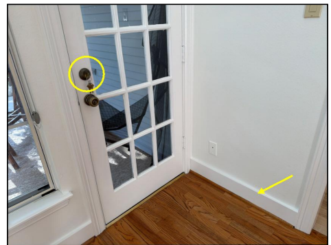
Family room exit doorstop noted to be missing/Keyless locks are required on exit doors
