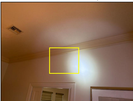
Poor quality drywall finish observed at the dining room wall
