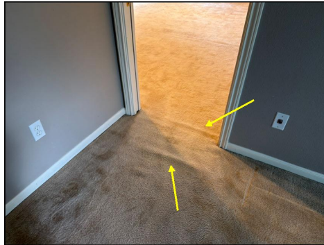
Loose carpet flooring observed at the garage apartment
