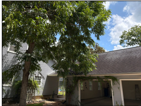
Tree branches should be cut back and kept clear of the roofing materials
