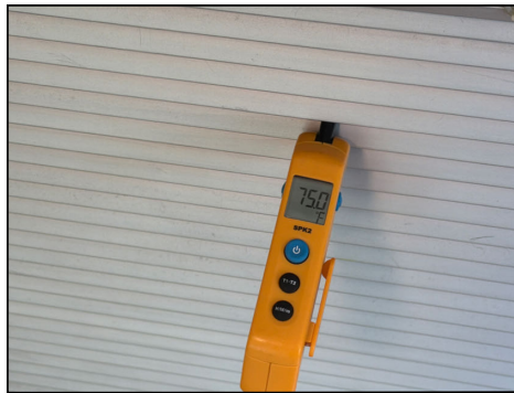
AC return air temperature/15-20 degree temperature differential is desired
