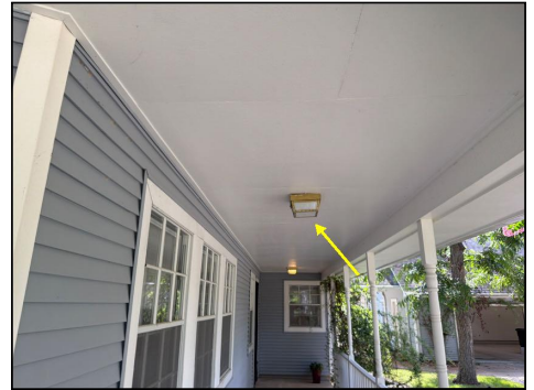
Exterior fixtures did not function at time of inspection
