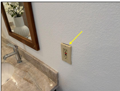
Primary bathroom outlet is not installed properly/loose cover plate
