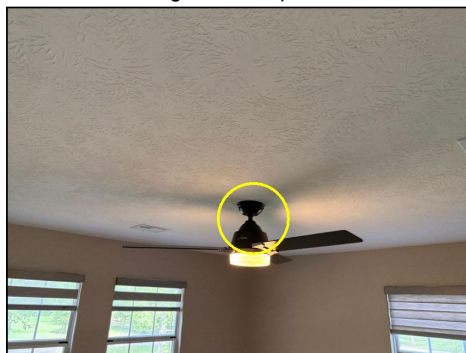
Unnecessary ceiling fan down rod observed in the front left secondary bedroom
