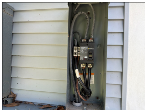
Panel appeared to be performing as intended
