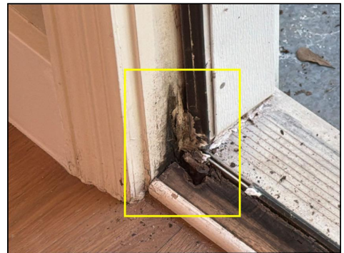
Front balcony door frame observed to be moisture damaged
