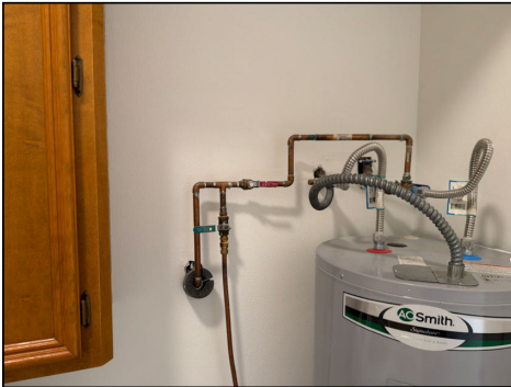
Unidentified supply lines observed at the water heater in the laundry area/Likely for water source AC system
