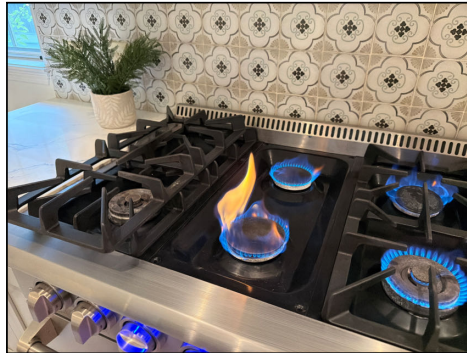
Range burners did not function properly/Did not appear to sit correctly
