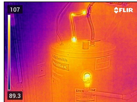
Water heater appeared to be performing as intended
