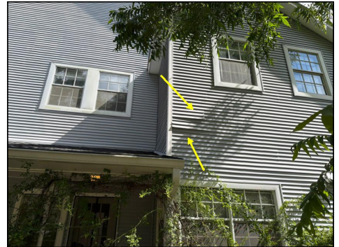
Damaged/loose siding observed on the right side of the home
