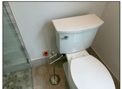
Upstairs right bathroom outlet is not GFCI protected
