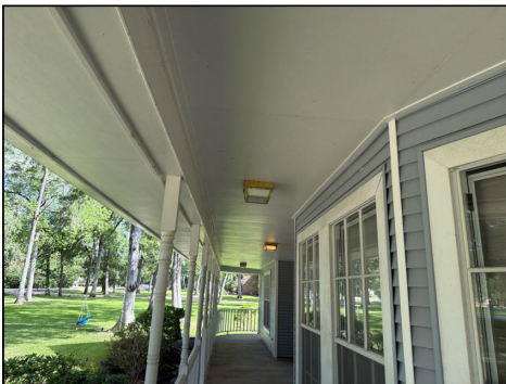
Exterior fixtures did not function at time of inspection
