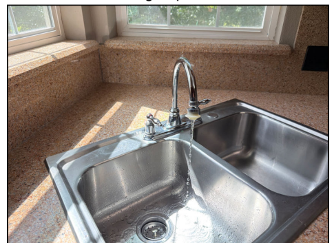
Low water pressure noted at the garage apartment fixtures
