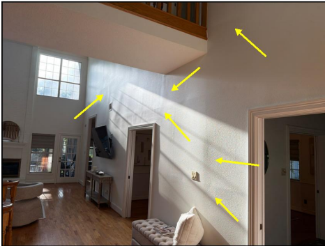
Nearly every drywall seam visible at the family room wall with bright sunlight illuminating
