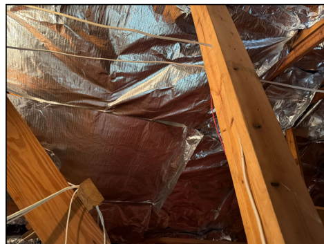
Foil sheets noted to be present in the attic/Attempt to create radiant barrier
