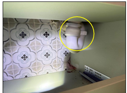
Accordion style/amateur drain observed in the half bathroom
