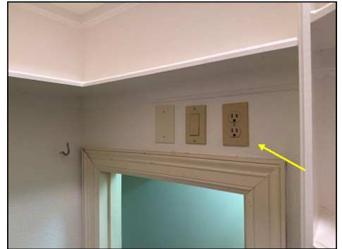
Out of ordinary outlet location observed inside the kitchen pantry
