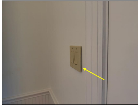
Dining area switches are not flush to the wall
