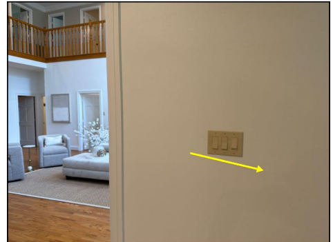
Crooked switches observed throughout the home
