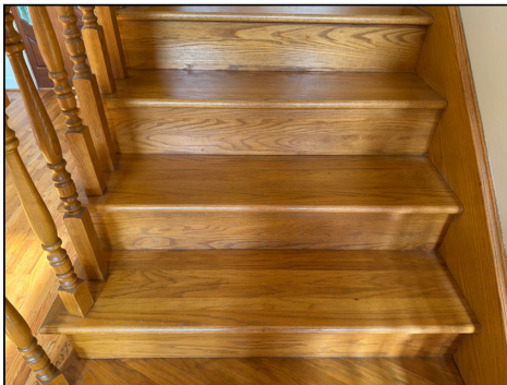
Typical squeaks and pops noted at the stairs
