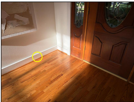
Front entry doorstop observed to be missing
