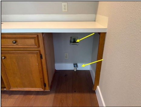
Plumbing for an ice machine noted to be present at the wet bar
