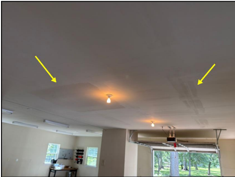
Inconsistent paint observed at the rear garage ceiling
