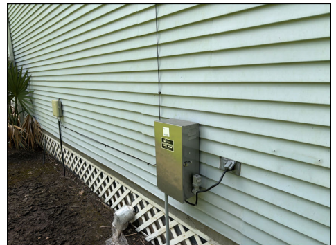
Exterior lighting and timers were not inspected
