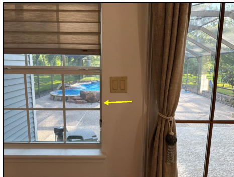
Primary bedroom switches observed to be crooked
