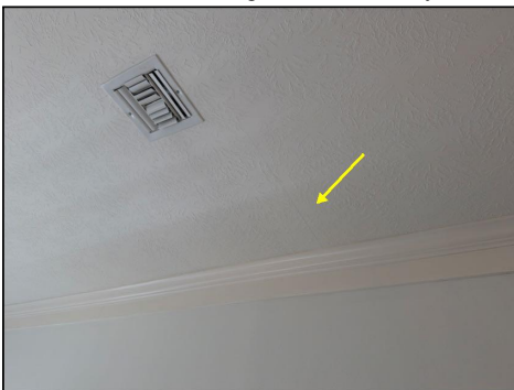
Drywall movement cracking observed at the primary bedroom ceiling
