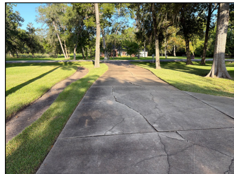
Multiple sections of the driveway observed to be cracked/broken
