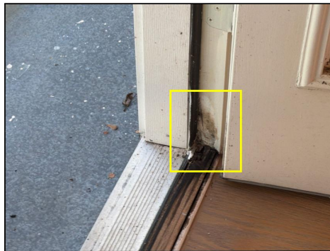
Front balcony door frame observed to be moisture damaged
