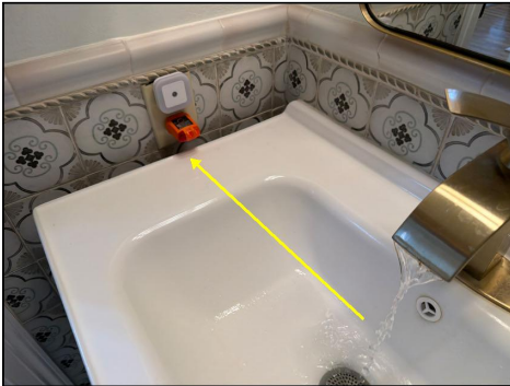
Half bathroom outlet is not GFCI protected
