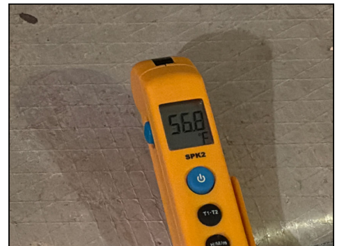
Garage AC supply temperature/Unit was cooling well at the time of inspection
