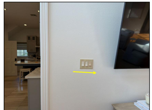
Family room switches observed to be crooked
