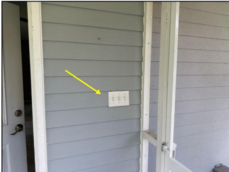
Exterior switch covers noted to be missing at the garage apartment
