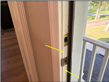
Front balcony door frame observed to be damaged/split
