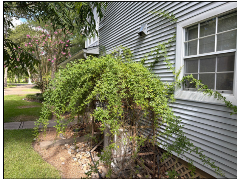
Foliage should be cut back and kept clear of the exterior walls
