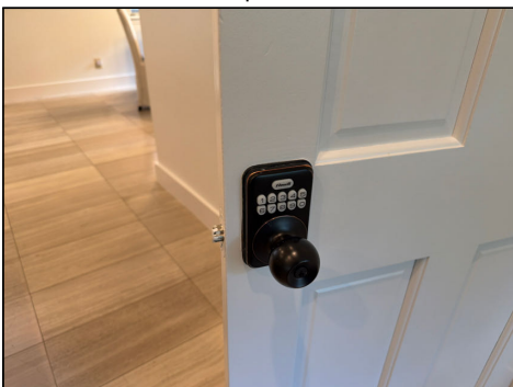
Out of ordinary key lock/combination door hardware observed at the kitchen pantry
