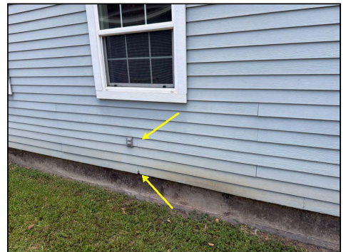
Damaged siding observed at the garage apartment
