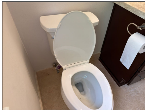
Upstairs front left commode was noted to be extremely slow to fill
