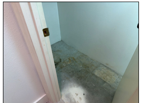
Flooring was not present at the closet under the rear stairs
