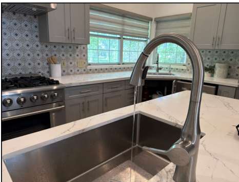
Hot and cold supply reversed at the island sink fixture
