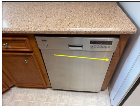
Garage apartment dishwasher is not installed square to opening
