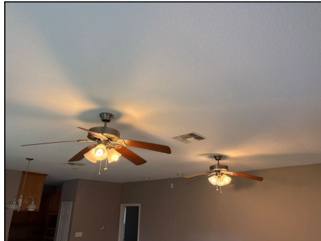
Drooping/weathered ceiling fan blades observed at the garage apartment
