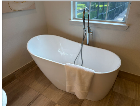
Primary bathtub is not installed properly/easily moves
