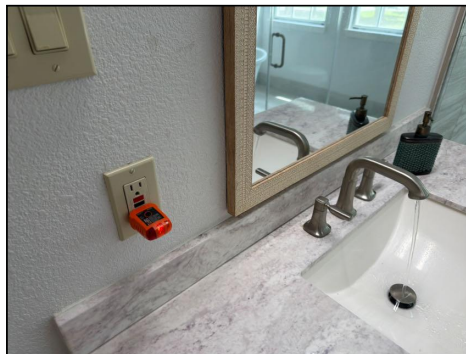
Upstairs right bathroom outlet shows ground reading/not GFCI protected
