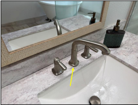
Upstairs, right vanity sink fixture is loose
