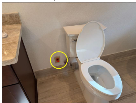
Primary bathroom outlet is not GFCI protected
