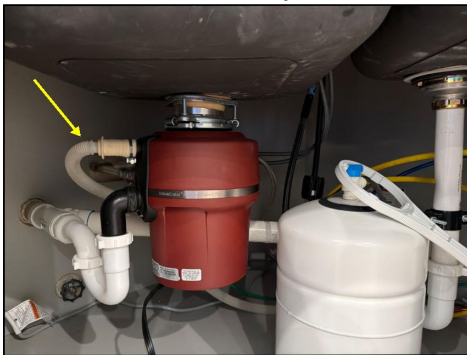
Air gap is missing at the dishwasher drain
