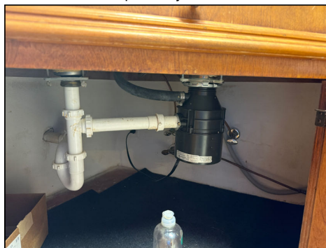
Disposal noted to be present at the garage apartment/typically not found with septic systems
