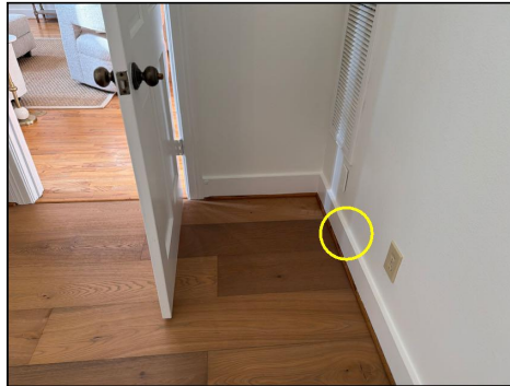
Primary bedroom doorstop noted to be missing
