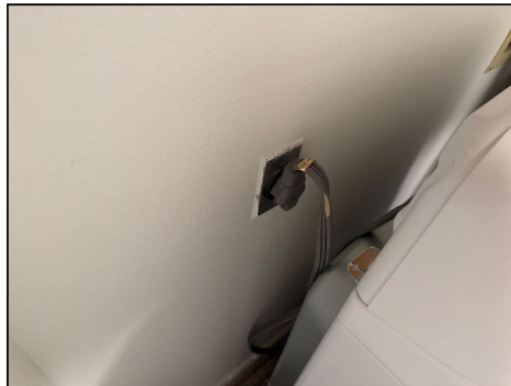
Electric dryer option noted to be present
