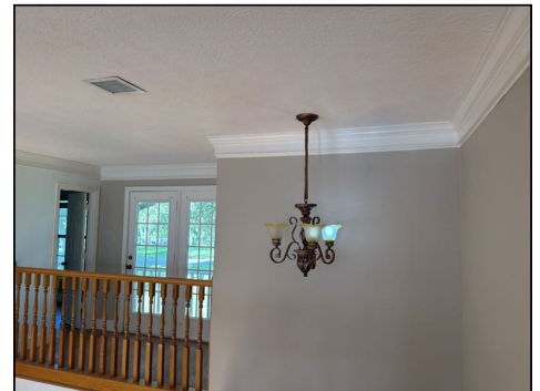
Fixture at the stairs did not function properly
