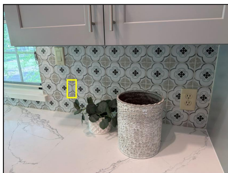
Spacing of the kitchen backsplash outlets does not meet current standards
