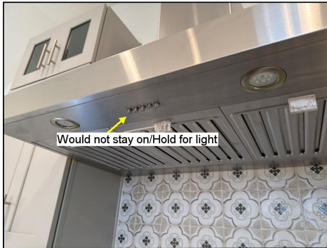
Button for the vent hood light did not function properly
