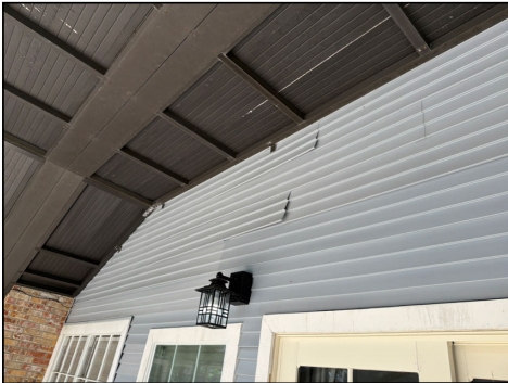
Loose/damaged siding noted at the rear of the home
