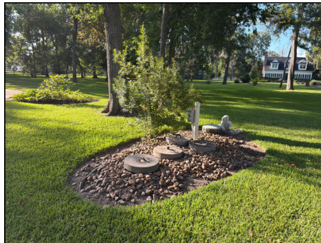
Septic equipment observed on the right side of the property
