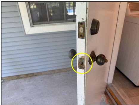
Laundry exit door hardware did not function properly
