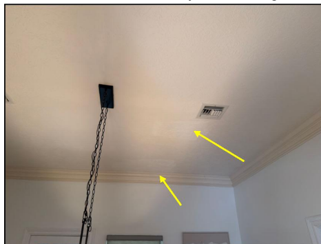
Inconsistent/incomplete paint observed at the dining room ceiling
