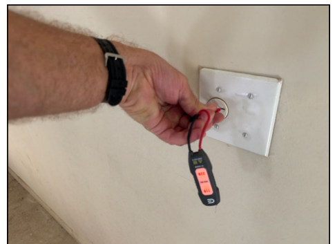
Rear 220 outlet in garage appeared to be performing as intended
