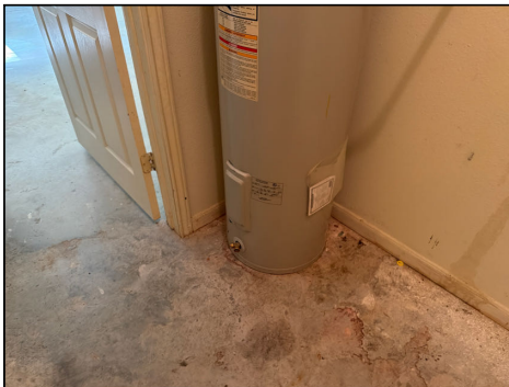
Overflow pan/drain line noted to be missing at the garage apartment unit
