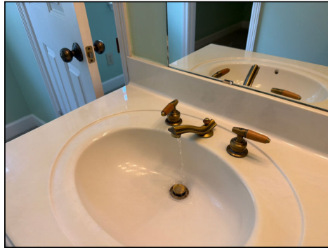
Substandard water pressure noted to be present throughout the home
