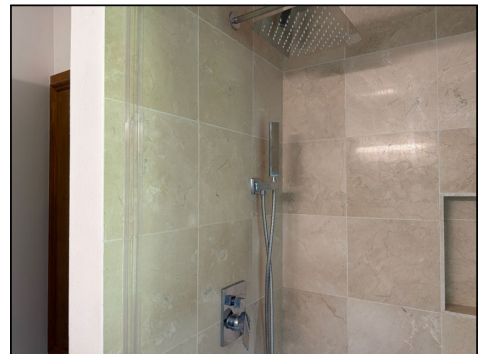
Upstairs front left secondary shower fixture did not function properly/Low pressure
