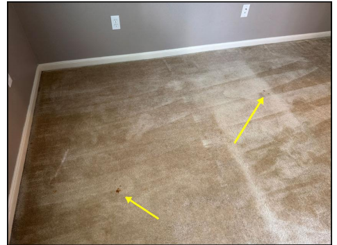
Garage apartment carpet flooring observed to be stained
