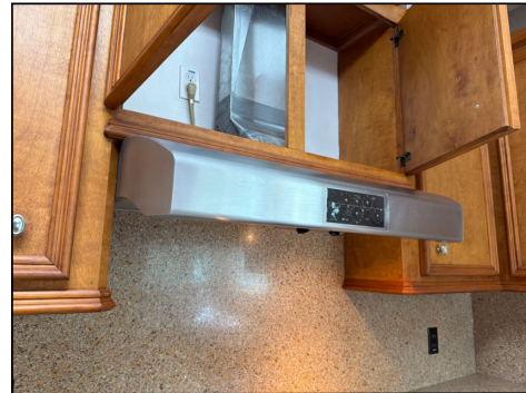
Garage apartment unit noted to be extremely noisy
