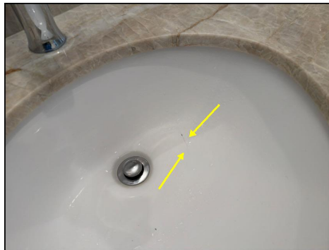
Primary vanity sink observed to be damaged/cracked
