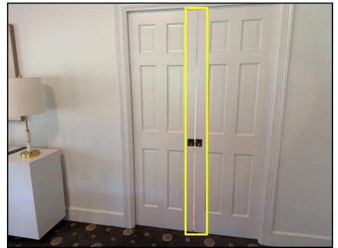
Inconsistent reveal observed at the formal living room pocket doors when closed
