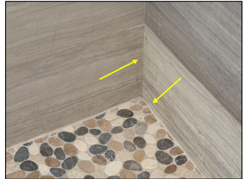
Cracked grout observed at the primary shower surround
