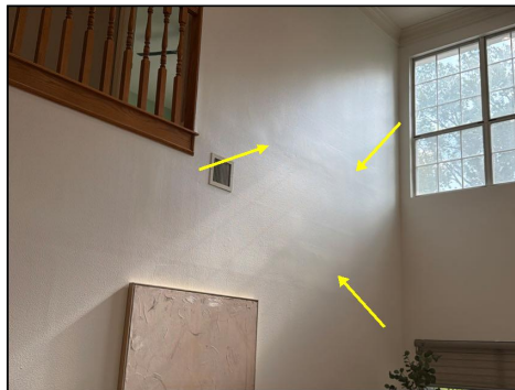
Poor quality drywall/texture finish observed at the family room high wall
