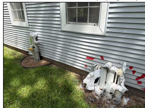
Deteriorated insulation observed on the right side of the garage
