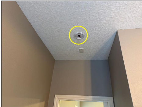
Garage apartment smoke alarm noted to be missing
