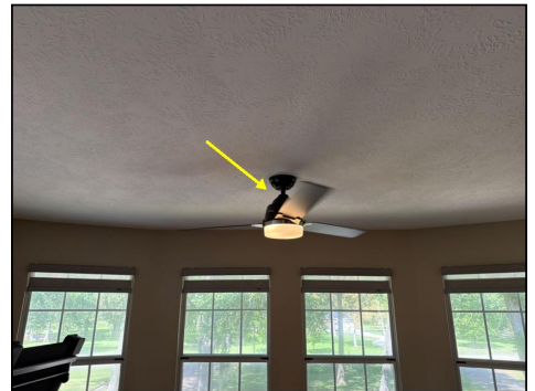
Unnecessary ceiling fan down rod noted at the front right game room/Eight foot ceiling should be flush mount
