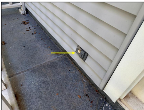
Broken outlet cover noted at the front balcony
