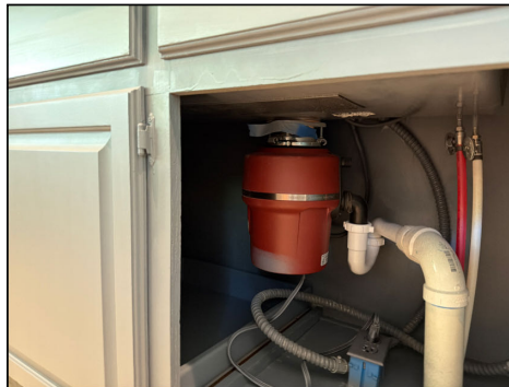
Island disposal did not function at time of inspection/jammed
