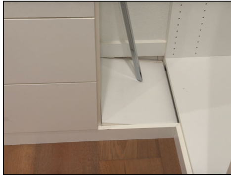
Damaged shelving observed in the primary closet
