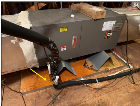
Evidence of previous secondary drain activity noted at the garage unit/Rusty overflow pan
