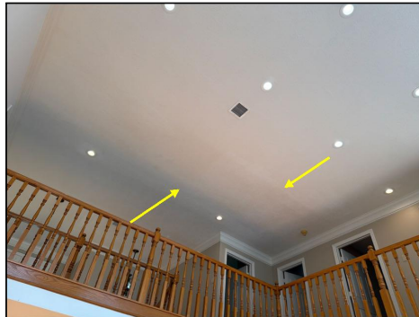
Evidence of previous repair/inconsistent finish observed at the family room ceiling
