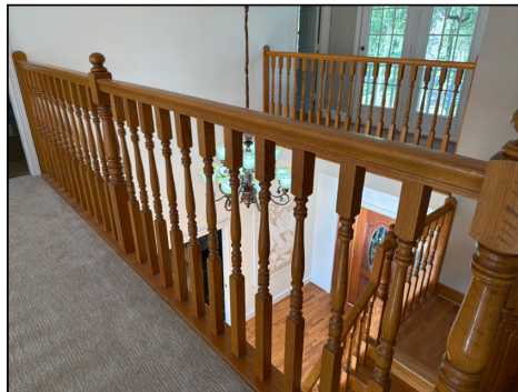
Baluster spacing does not meet current standards
