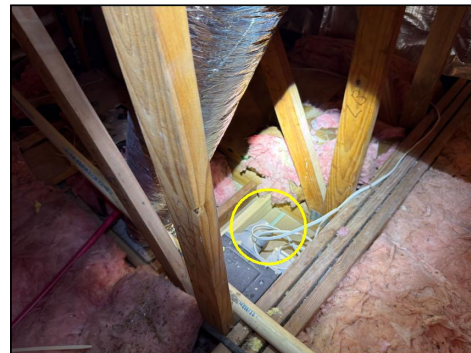
Upstairs right bathroom fan noted to terminate in the attic
