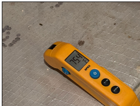
Garage AC return air temperature/15-20 degree temperature differential is desired
