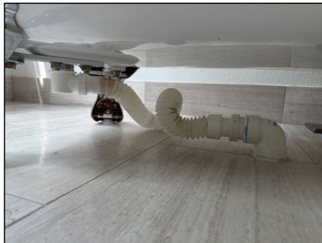
Amateur/improper drain installation at the upstairs right tub
