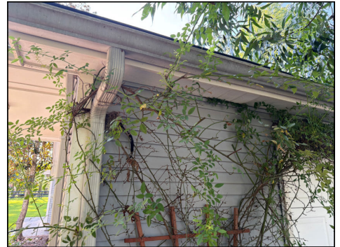
Damaged exterior paint finish from foliage growth observed
