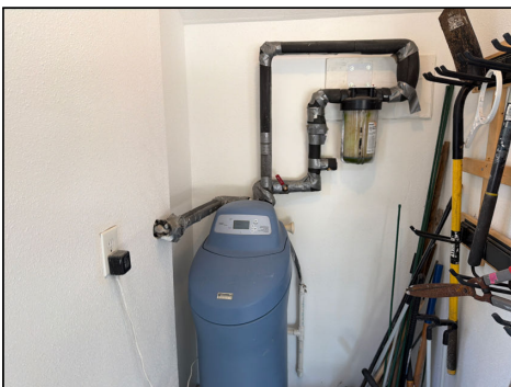
Water softening system was not inspected
