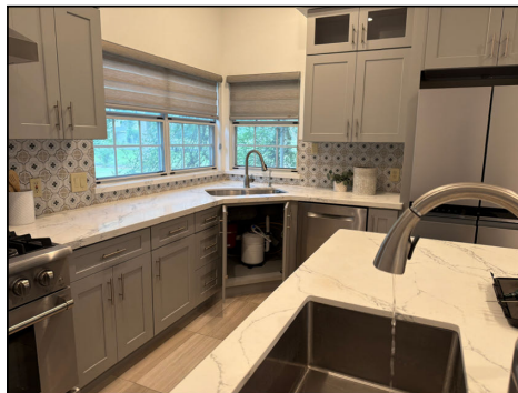
Water pressure down to trickle at some times during inspection
