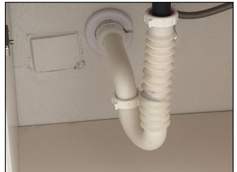
Amateur/improper drain installation at the upstairs right vanity sink
