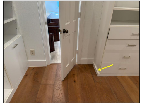
Primary closet doorstop noted to be missing
