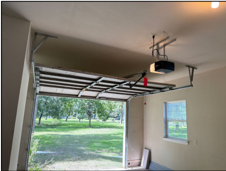
Rear door opener did not function properly/button had to be held to close
