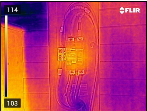
Panel appeared to be performing as intended
