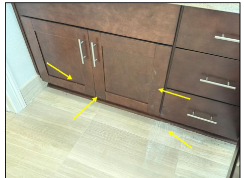
What appeared to be grout residue observed on the primary bathroom cabinets
